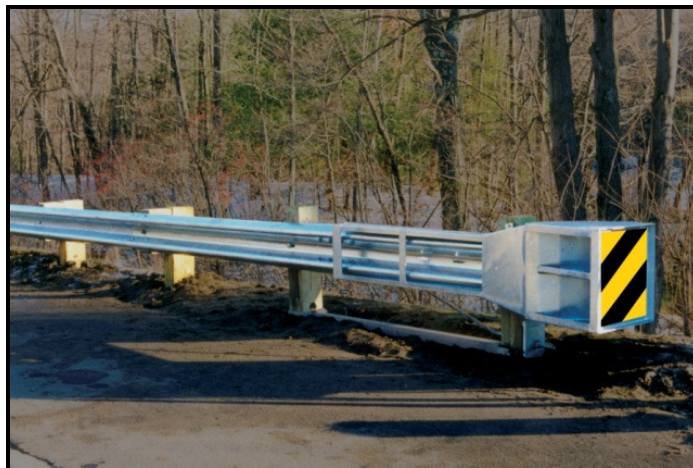
Figure 11: A Midwest non-proprietary energy-absorption terminal
