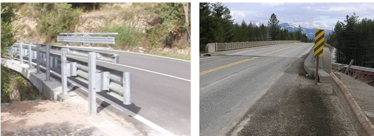
Figure 53: Examples of hazardous safety barrier terminations
