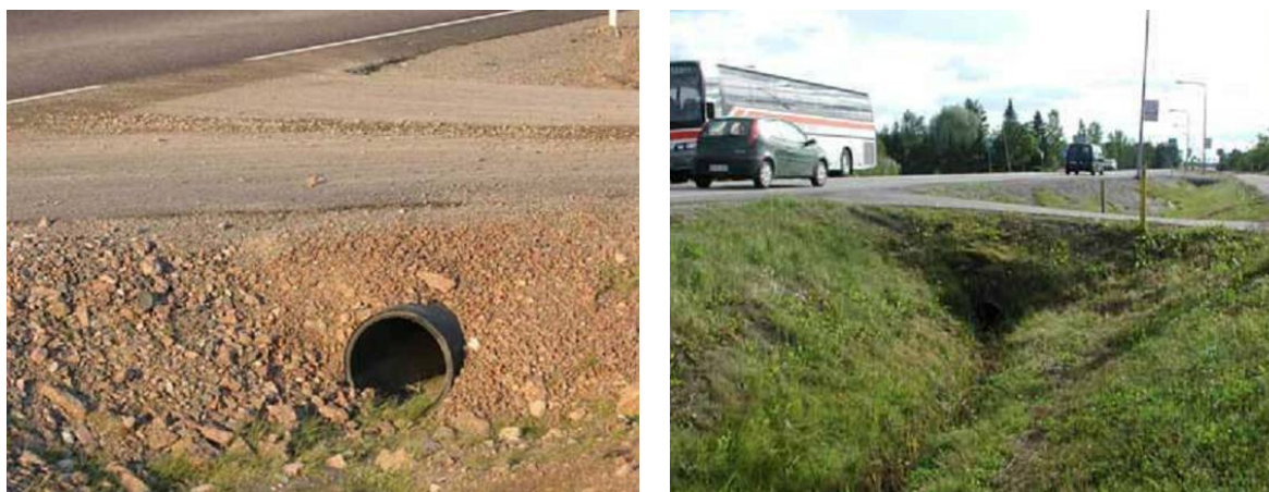
Figure 55: Examples of hazardous drainage features (Source: [A.2])
