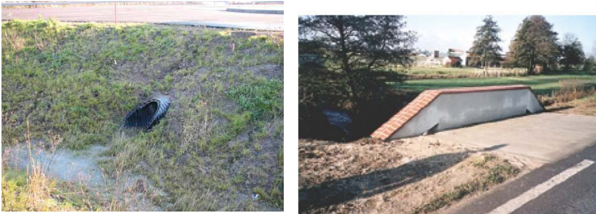
Figure 72: A bevelled culvert end ( left ) and a chamfered parapet ( right ) (Sources: [A.2], [A.27])
